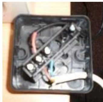
Figure 16 Interior of a Junction Box
