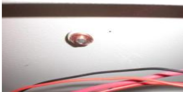
FIGURE 2 EARTH BOLT REMOVED
